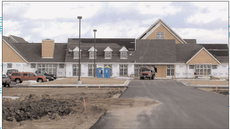
Middleton Community Church is nearing completion, with Pozzi Wood Windows in place. Designed by Melissa Turk, the project is being built by Vogel Brothers.
